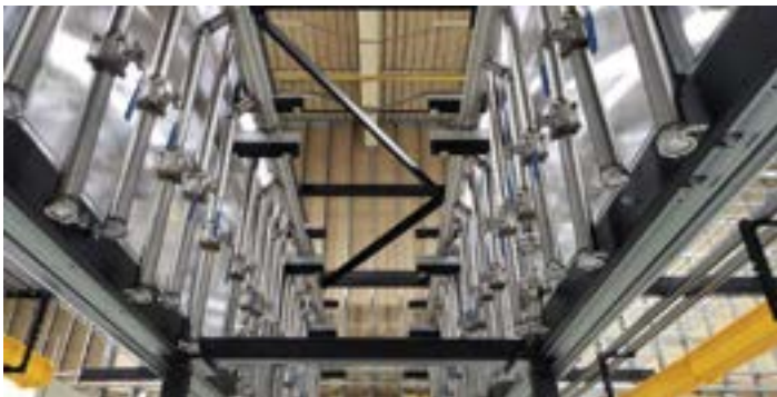
The HAC supports the integration of liquid cooling manifolds to cool high-density server racks.
